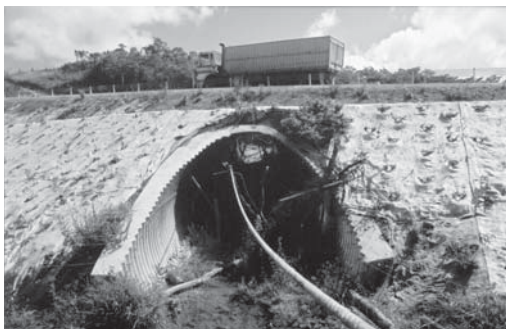
Faunal underpass, East Evelyn Road. (Photo: Jonathon Munro)
